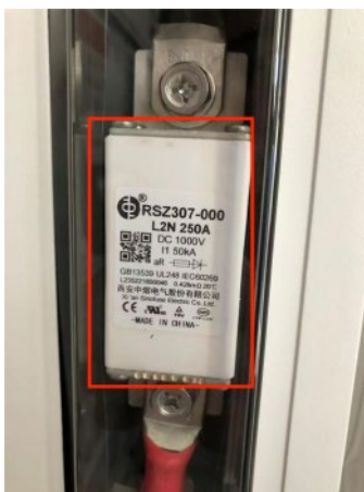
Figure 18 – battery cluster fuse
