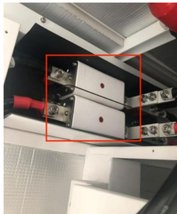
Figure 17 - main circuit fuses
