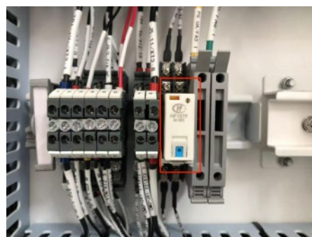
Figure 32 – exhausts fan test button
