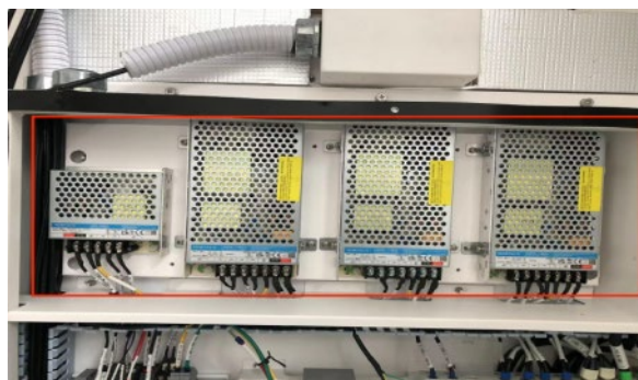
Figure 35 – switching power supply
