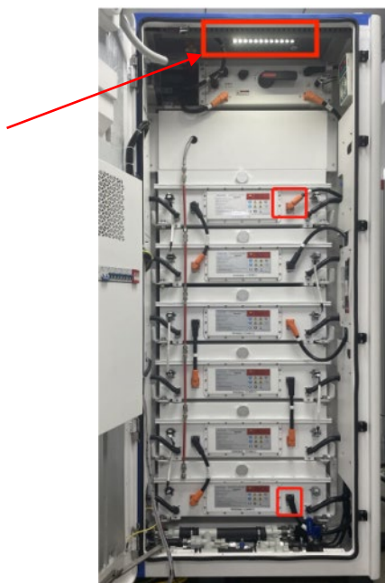
Figure 28 - internal illumination strip
