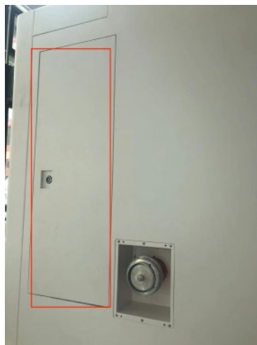
Figure 43 – Fire extinguisher cylinder access door
