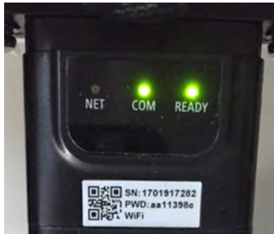
Figure 91 - Irregular communication status between the adapter and remote server
