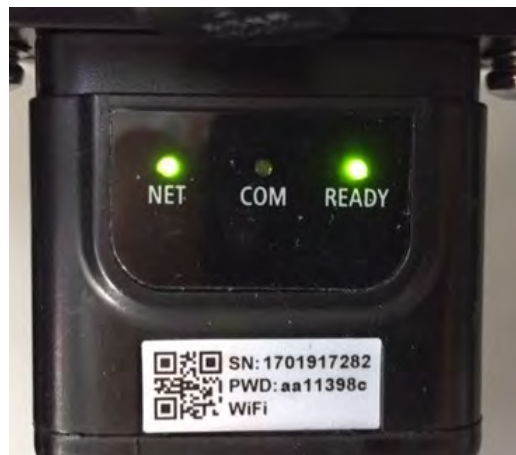
Figure 90 - Irregular communication status between the inverter and adapter
