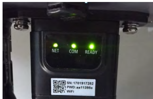
Figure 95 - Final status of LEDs
