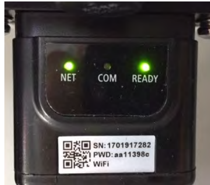
Figure 96 - Irregular communication status between inverter and adapter
