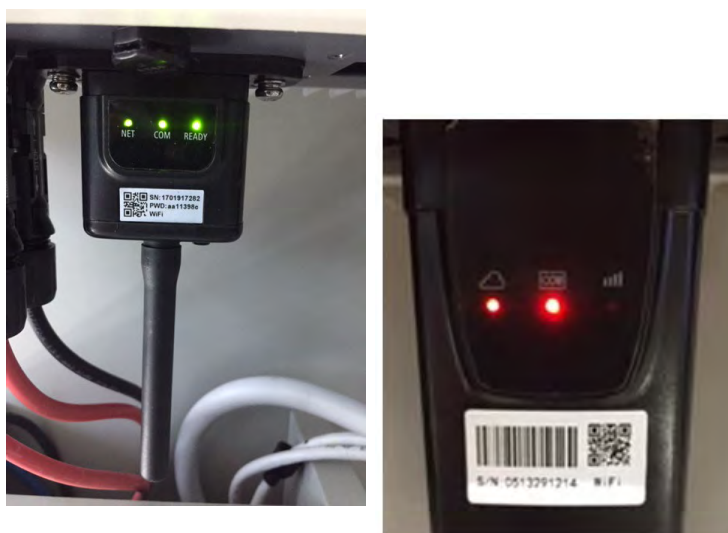
Figure 77 - Final status of LEDs
