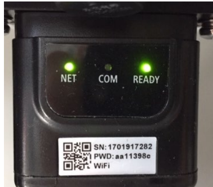
Figure 150 - Irregular communication status between inverter and adapter
