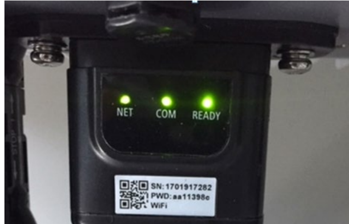
Figure 143 - Final status of LEDs
