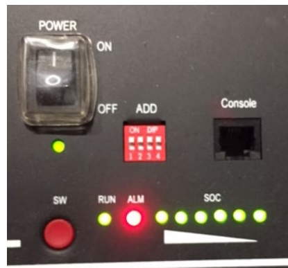
Figure 111 - Battery status after setting the POWER switch to ON and pressing the SW button
