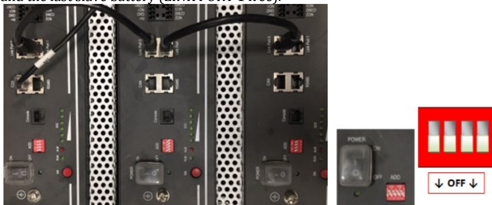
Figure 16- Connecting the communication cable between three Pylontech batteries
