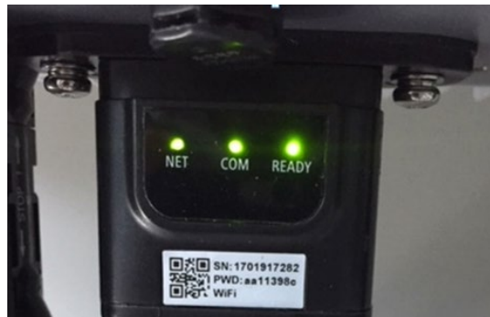
Figure 149 - Final status of LEDs
