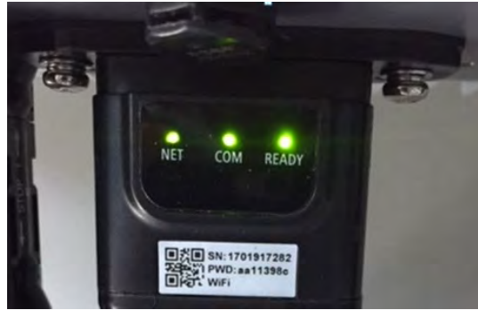
Figure 69 – Final status of LEDs
