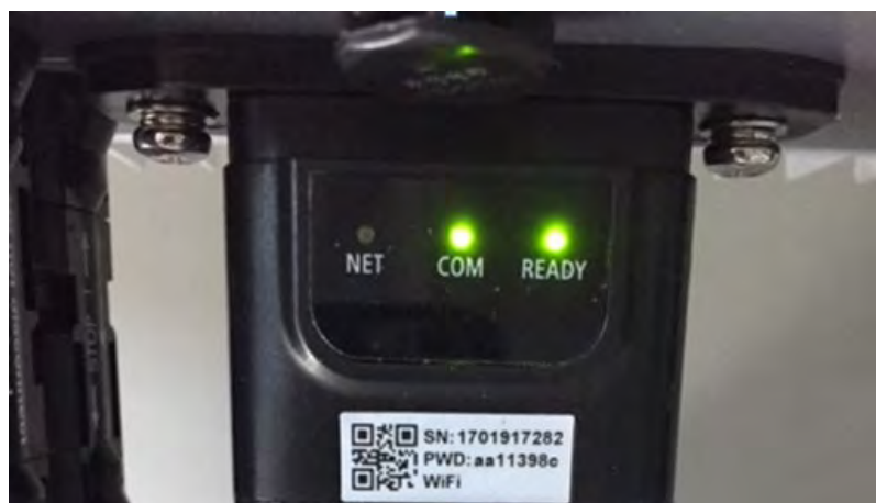
Figure 62 – Initial status of LEDs
