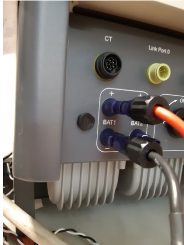
Figure 130 - Inverter-side DC power connection with a single battery input populated
