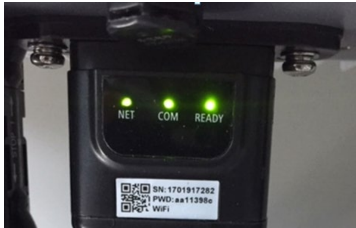
Figure 243 - Final status of LEDs
