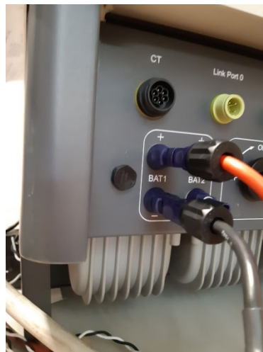
Figure 164 - Inverter-side DC power connection with a single battery input populated
