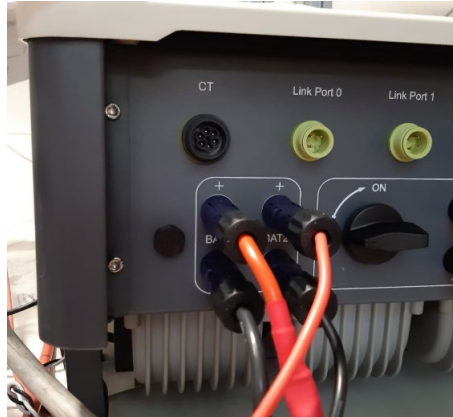
Figure 64 - Inverter-side DC power connection with two battery inputs populated
