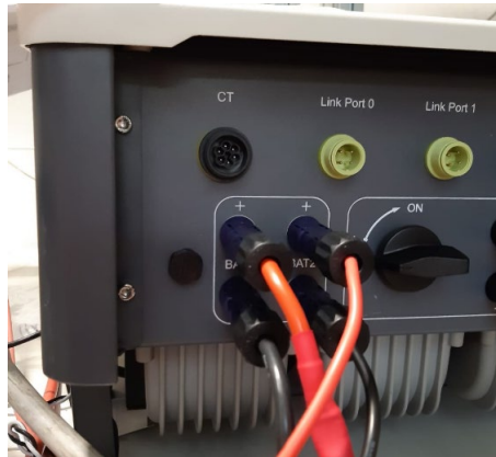
Figure 111 - Inverter-side DC power connection with two battery inputs populated
