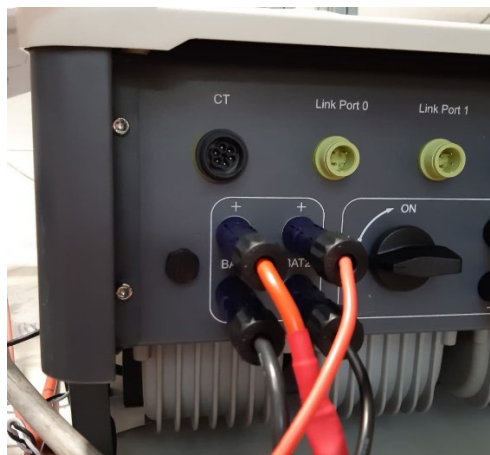
Figure 78 - Inverter-side DC power connection with two battery inputs populated
