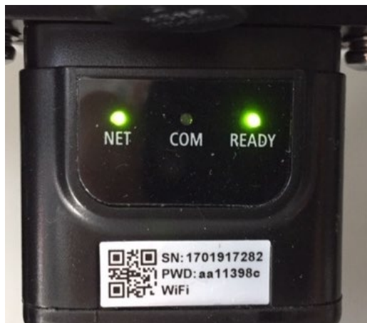
Figure 244 - Irregular communication status between inverter and adapter
