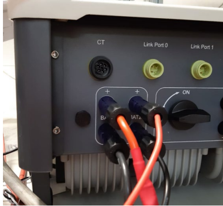
Figure 56 - Inverter-side DC power connection with two battery inputs populated
