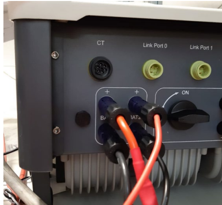
Figure 148 - Inverter-side DC power connection with two battery inputs populated
