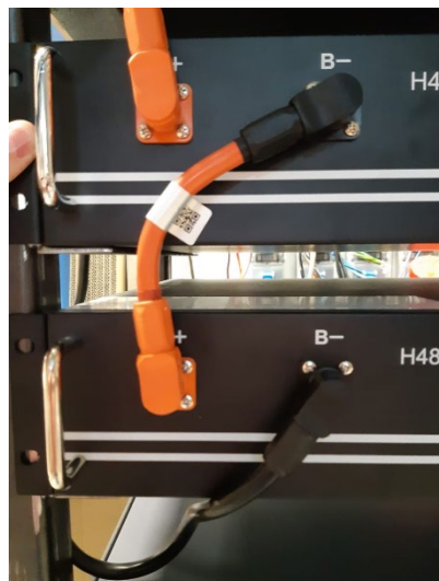
Figure 45 - Power connection (negative) between the BMS and the last battery module
