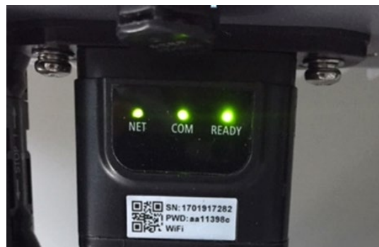
Figure 249 - Final status of LEDs
