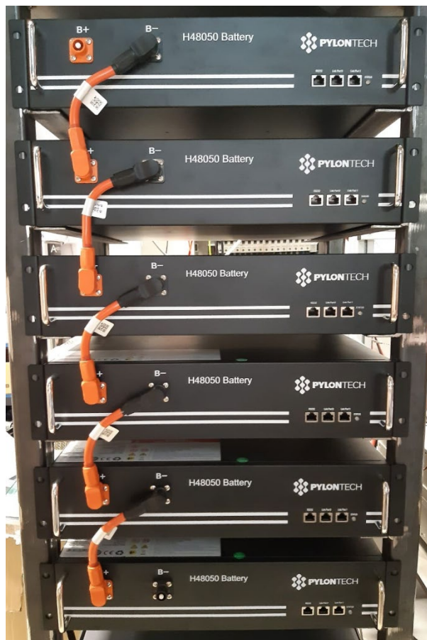
Figure 42 - Power cable between battery modules
