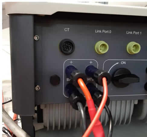
Figure 101 - Inverter-side DC power connection with two battery inputs populated
