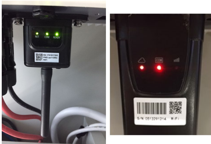
Figure 231 - Final status of LEDs
