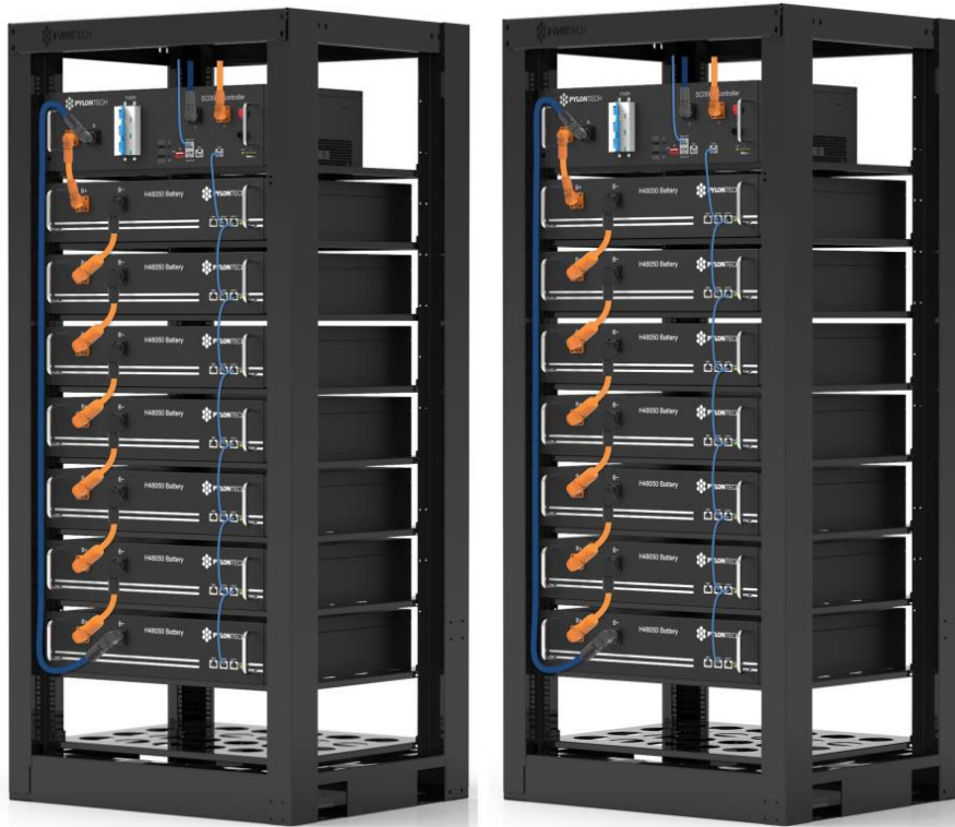
Figure 49 - Two battery towers
